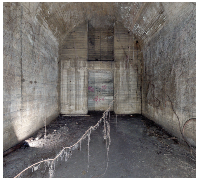
World War II reinforced-concrete baffle wall in a single-track tunnel south of St James Station in 2019 (Image courtesy of BeThere for Sydney Trains).
