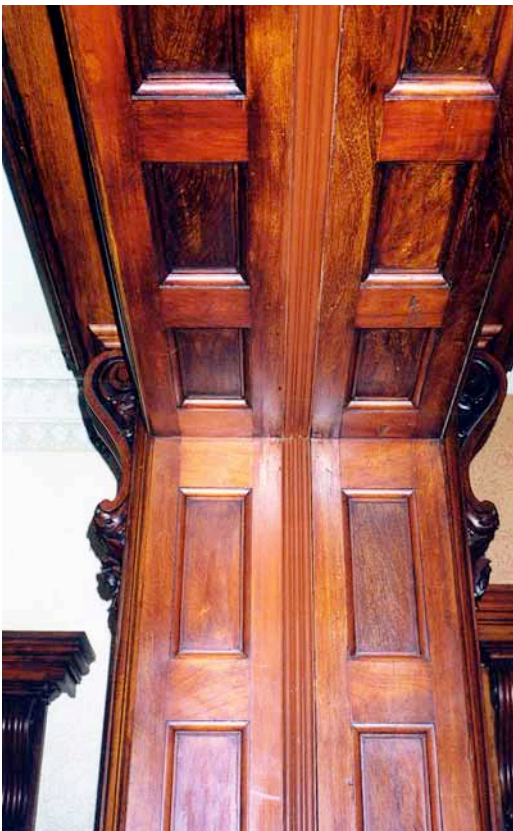
FIGURE 2.44: Detail of doorcase dividing the parlour from the dining room, showing the recent filing of the sliding door gap.
