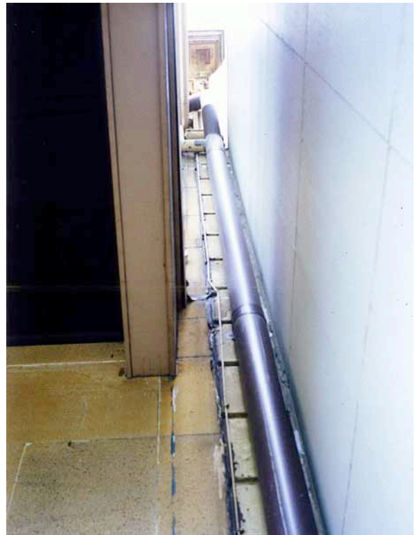
FIGURE 2.30: Surviving wall section behind downpipe, from No. 131 Macquarie Street to the north
