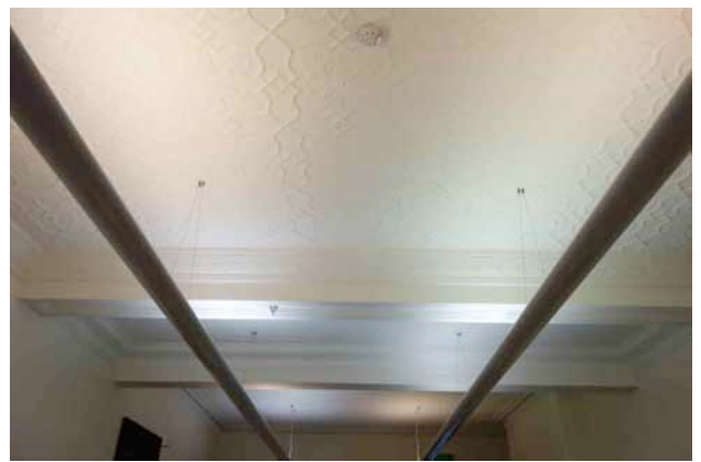
FIGURE 2.54: Ceiling detail to the main office on the second floor looking west
