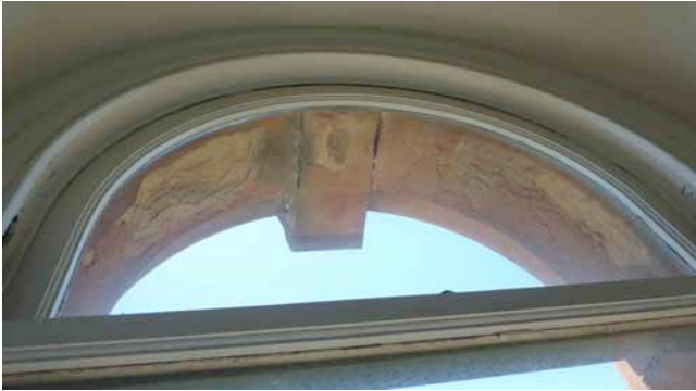
FIGURE 2.59 Delamination of stonework above attic windows
